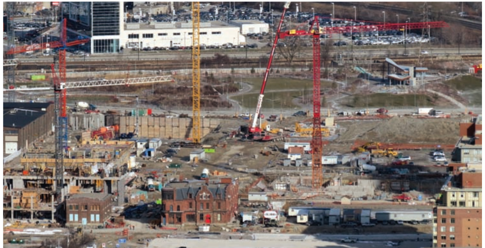
Aerial view of current construction of the Toronto 2015 Pan Am/Parapan Am Games' Athletes' Village located in the West Donlands in the newly-named Canary District.
